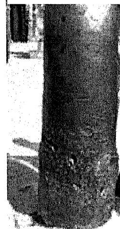
Damage by corrosion ne
